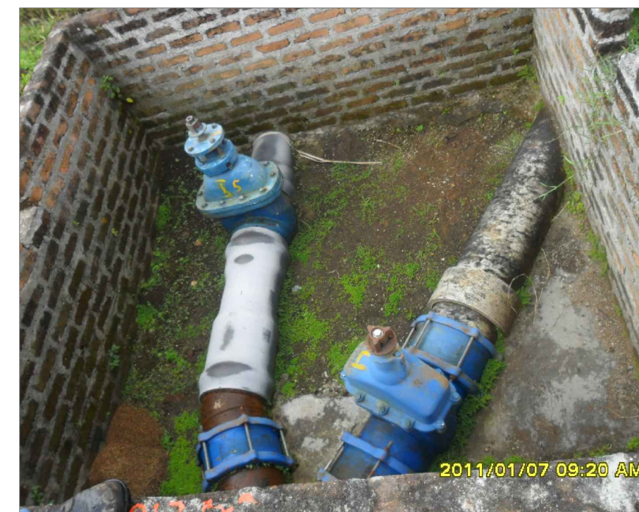
VISTA CAJA BYPASS
