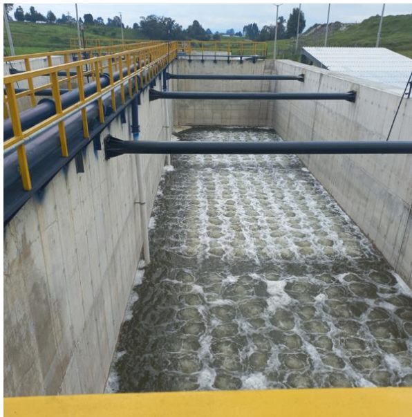
Illustration No. 33: Aeration tank performance test – Jan 2024, Facatativá
