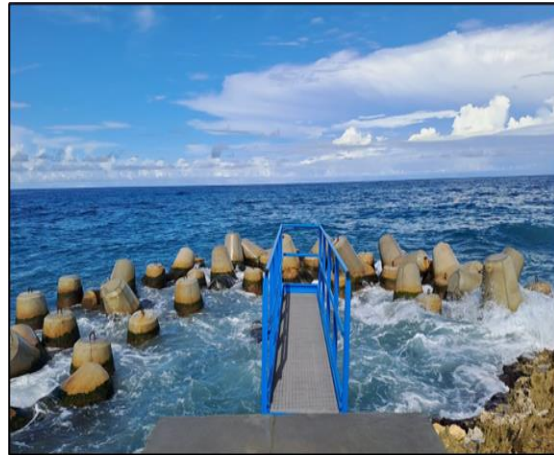
Seawater intake system via direct pumping
