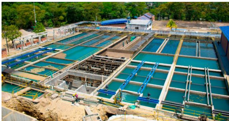
Illustration No. 46: Modernization of the La Esmeralda Drinking Water Treatment Plant DWTP and Implementation of the Water Loss Recovery Plan
