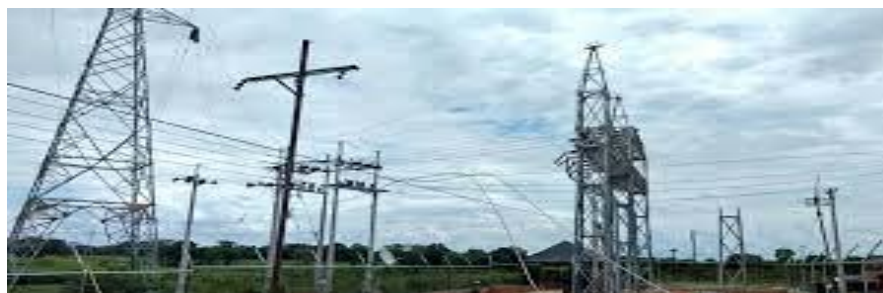
Illustration No. 47: Tibú - César Substation
