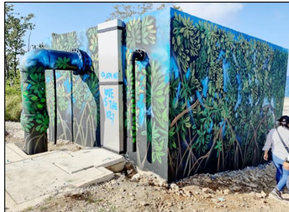
Pumping station for direct seawater intake.
